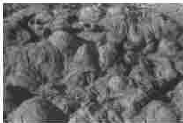
Fig 6.4 : Exfoliation (Flaking) and granular disintegration.
